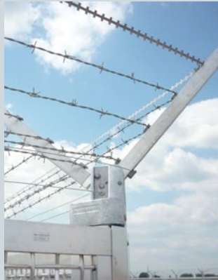
Barbed wire and Y-arm climbover protection
